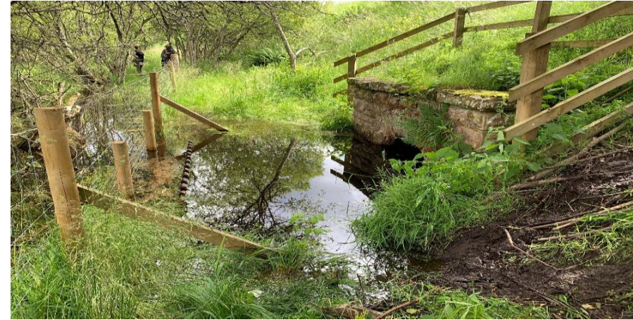
Flood waters around the culvert
